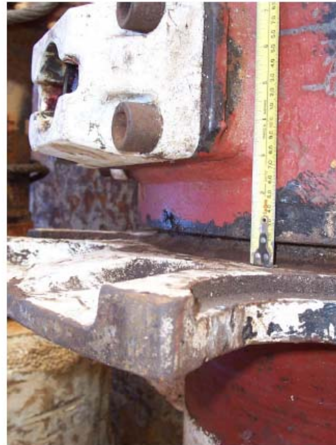
Figure 4. Gap Between MR6 Lift Sub & Riser Pin Flange
