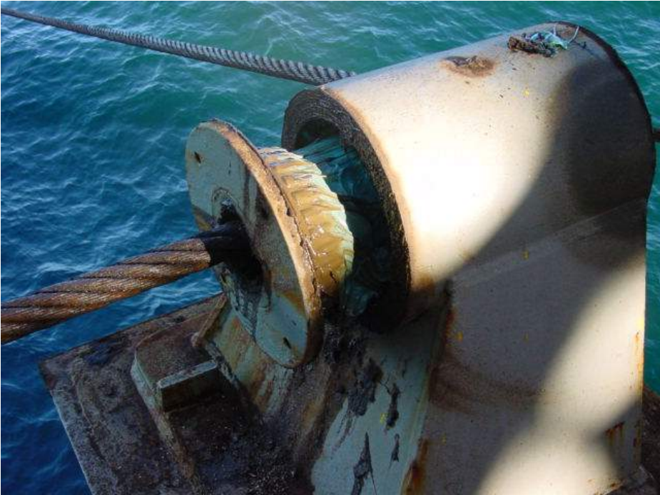
Port Fairlead Post Incident
