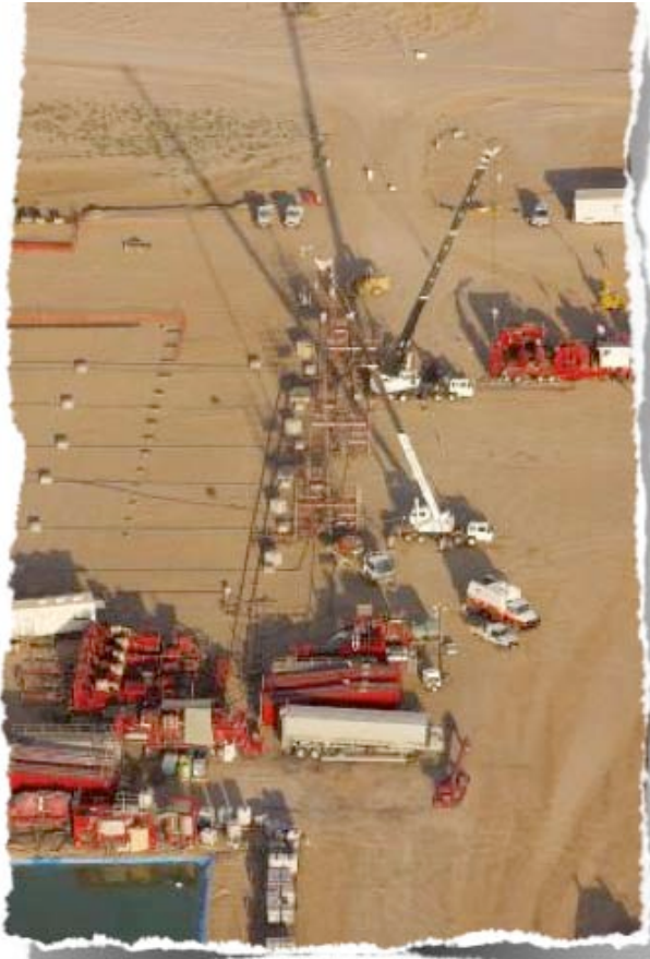
SimOps in Operation
